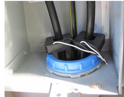
Split-Core CT's installed
